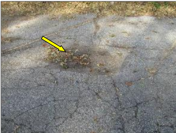
View of a depression in the asphalt paved parking area noted at the west portion of the Site.
