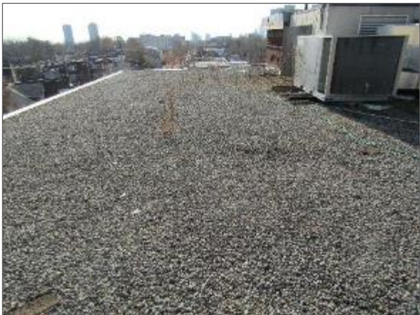
General view of the BUR system serving the Phase 3 (i.e., east) portion of the Site Building.
