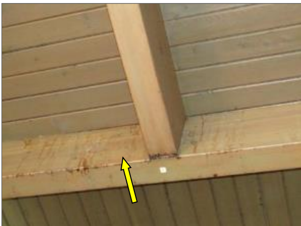
View of a roof leak through the modified bitumen roof system into the Grand Hall foyer noted within the Phase 2 portion of the Site Building.
