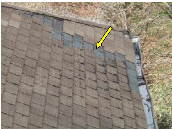
View of the missing asphalt shingles noted at the northwest portion of the sloped asphalt shingled roof system serving the Phase 1 portion of Site Building.
