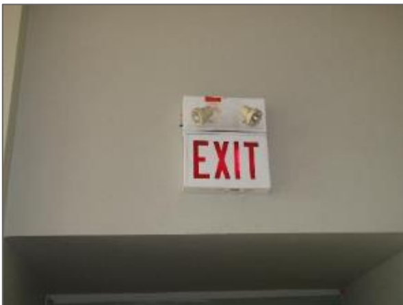
View of the typical illuminated exit signage and emergency lighting noted throughout the Site Building.
