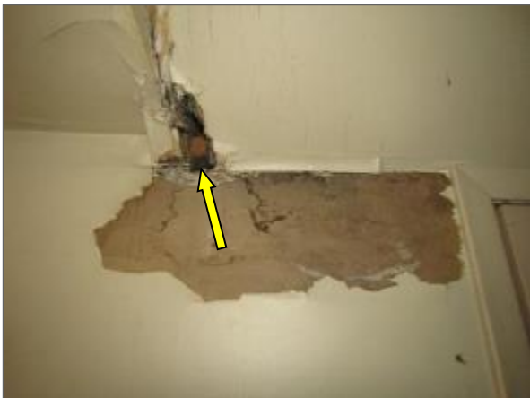
View of an active roof leak noted at the vicinity of the tower portion of Phase 1.
