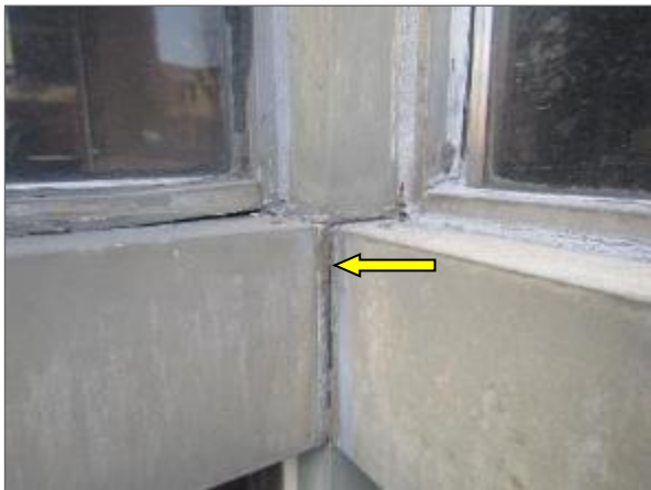
View of cracked perimeter window sealant noted on the south elevation of the Phase 3 portion of the Site Building.
