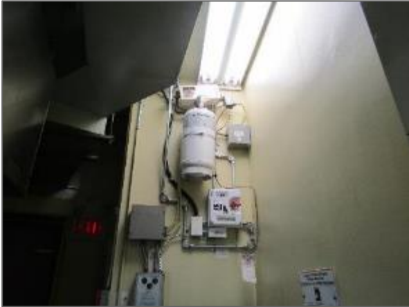
View of the fire suppression equipment noted within the kitchen.
