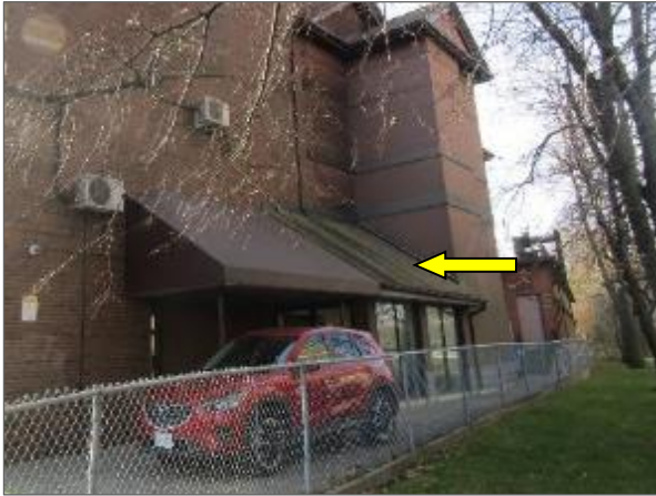
General view of the lower sloped asphalt-shingled roof system serving the Phase 4 (i.e., northeast) portion of the Site Building.
