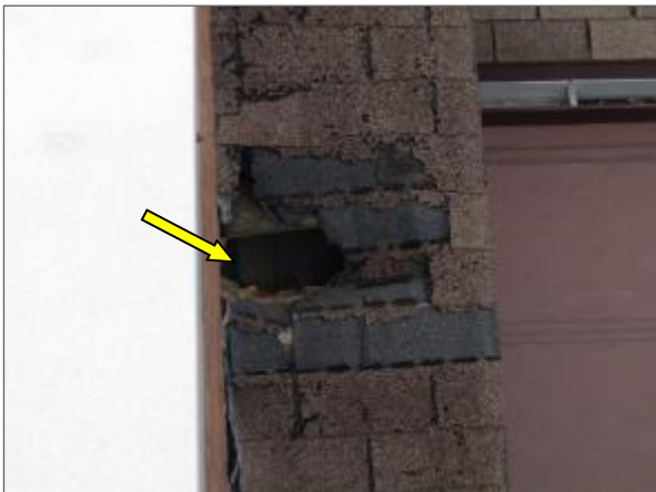
View of a hole through the sloped asphalt roof system noted at the north portion of the Phase 1 portion of the Site Building.
