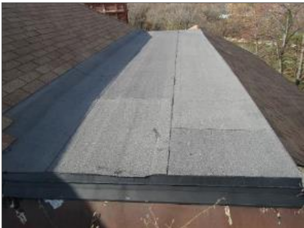
General view of the modified bitumen roof system noted atop the north-central portion of the Phase 1 portion of the Site Building.
