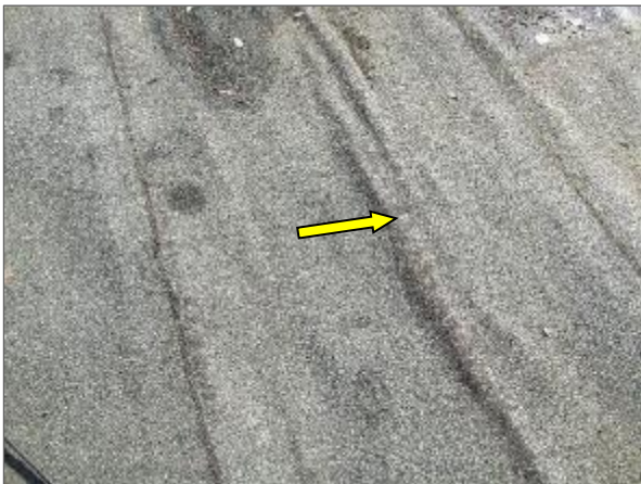
View of wrinkling of the modified bitumen membrane noted at the southeast portion of the modified bitumen roof system serving the Phase 2 portion of the Site Building.
