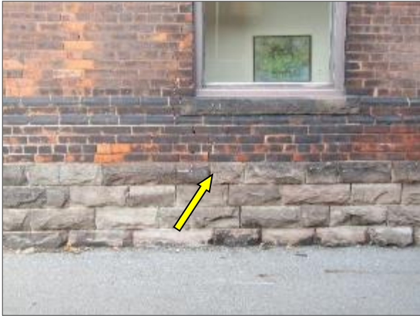
View of step cracking in the multi-wythe brick masonry and architectural block masonry wall noted on the south elevation of the Phase 1 portion of the Site Building.
