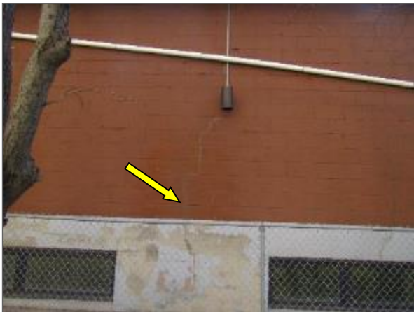
View of a vertical crack on the concrete block masonry wall noted on the north elevation of the Phase 2 portion of the Site Building.
