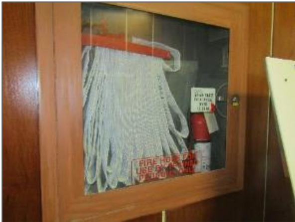
View of a typical fire hose cabinet complete with fire extinguisher noted in the east portion of the Site Building.
