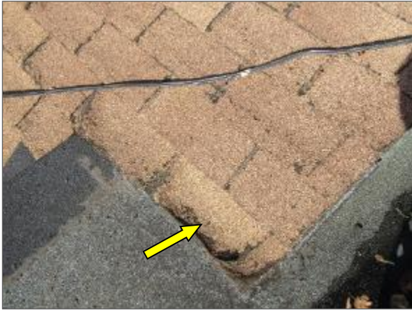
View of the typical worn/aged asphalt roof shingles serving the Phase 2 portion of the Site Building.
