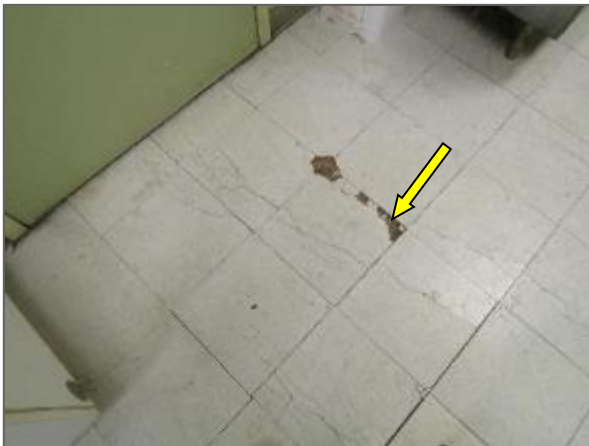
View of the cracked/deteriorated vinyl floor tiles noted in the kitchen area of the Phase 2 portion of the Site Building.
