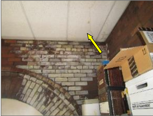
View of the water stained ceiling tiles and brick masonry noted within the tower of the Phase 1 portion of the Site Building.
