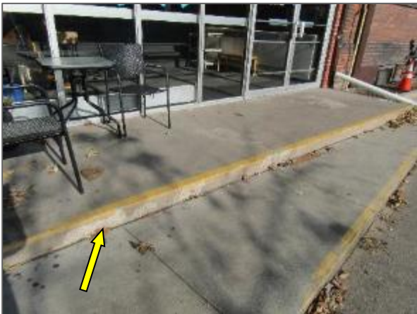
View of the spalled cast-in-place concrete walkway noted adjacent to the south elevation of the Site Building.
