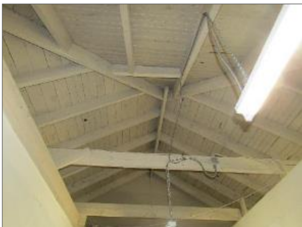
General view of the wood roof joists and decking noted within the gun range of the Phase 1 portion of the Site Building.
