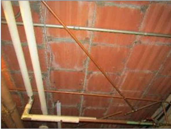
General view of the flat arch slab construction noted within the basement level of the Phase 2 portion of the Site Building.
