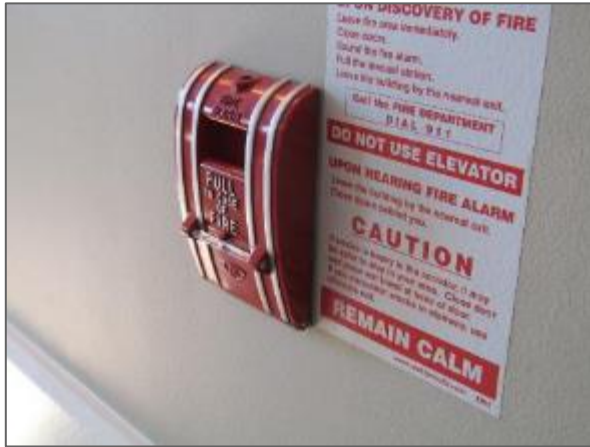
View of a typical manual pull station noted at strategic locations throughout the Site Building.
