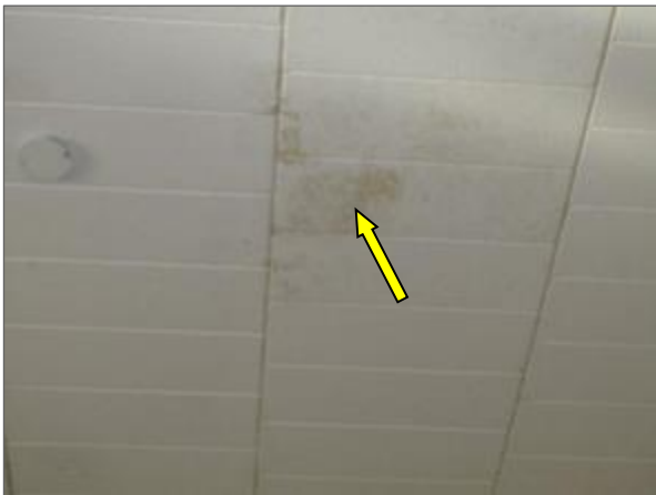
View of moisture staining on the underside of the concrete panel roof deck (i.e., indicating a previous roof leak) noted within the "Youth Room" on the top floor of the Phase 3 portion of the Site Building.
