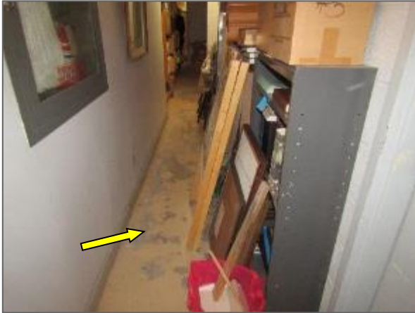
View of the deteriorated epoxy finished floor slab noted in the basement level of the Phase 3 portion of the Site Building.
