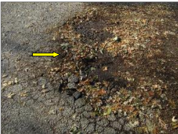
View of the deteriorated asphalt pavement noted at the west portion of the Site.
