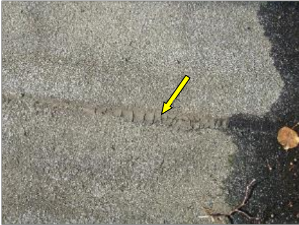
View of the typical cracked seals and worn/aged modified bitumen membrane serving the flat roof areas of Phase 2.
