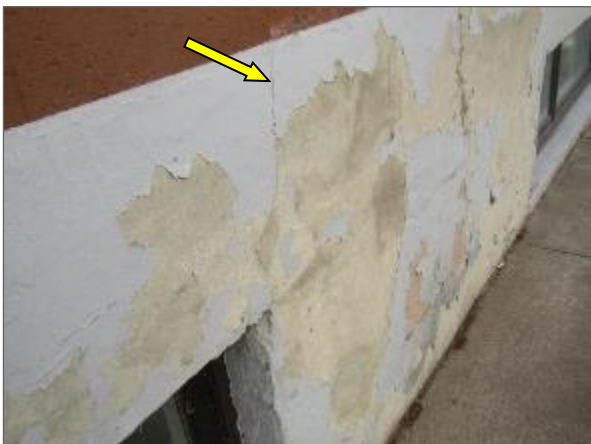
View of the cracked cement parging and peeling paint noted on the north elevation of the Phase 2 portion of the Site Building.
