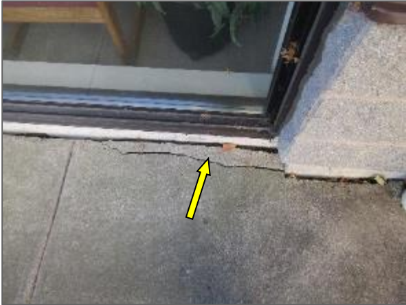
View of a crack in the cast-in-place concrete walkway noted adjacent to the north elevation of the Site Building.
