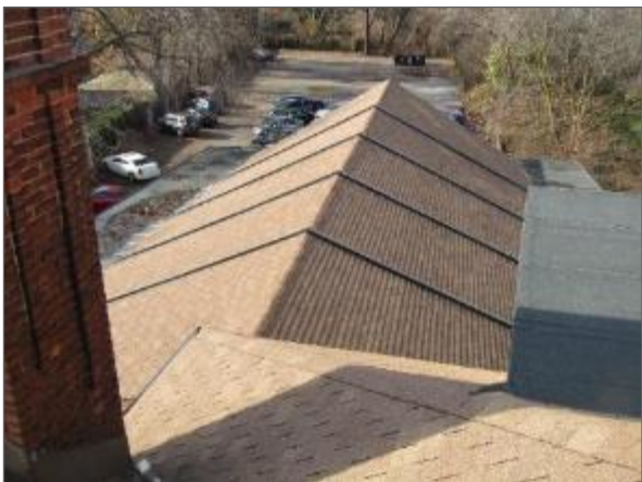
General view of the sloped asphalt roof system serving the Phase 2 (i.e., west) portion of the Site Building.
