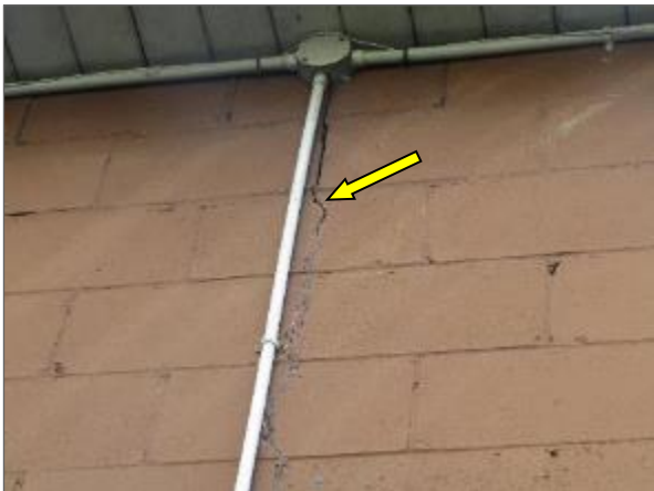
View of a vertical crack on the concrete block masonry wall noted on the north elevation of the Phase 2 portion of the Site Building.
