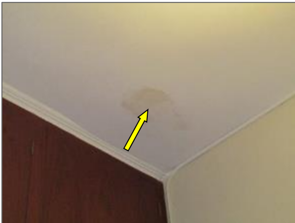
View of the water stained gypsum ceiling noted in a corridor of the Phase 3 portion of the Site Building.
