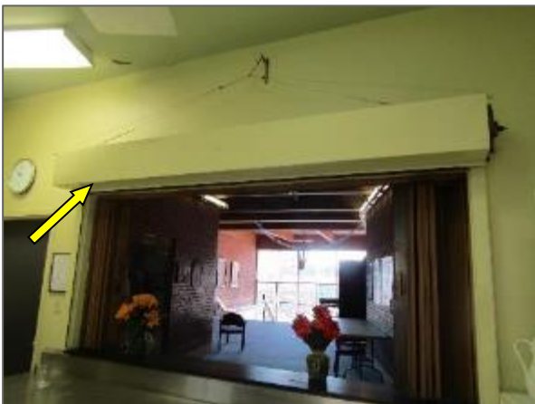
View of the fire shutter noted within the main kitchen area.
