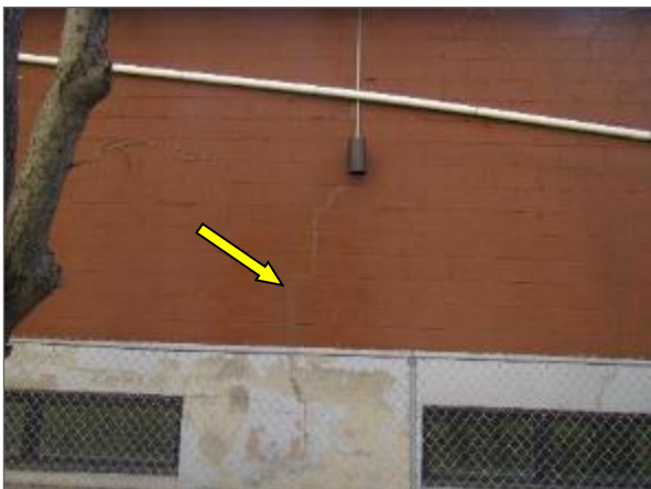
View of a vertical crack on the concrete block masonry wall noted on the north elevation of the Phase 2 portion of the Site Building.
