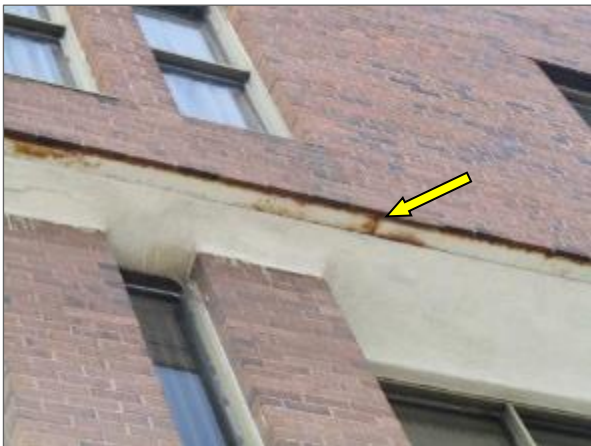
View of the corrosion on the steel beam noted on the east elevation of the Phase 3 portion of the Site Building.
