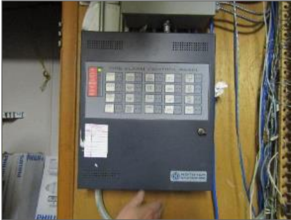
View of the fire alarm control panel noted in the basement level electrical room.
