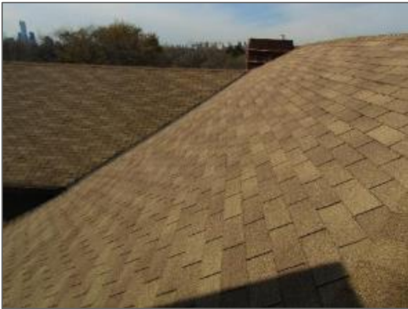
General view of the sloped asphalt-shingled roof system noted atop the Phase 1 (i.e., central) portion of the Site Building.
