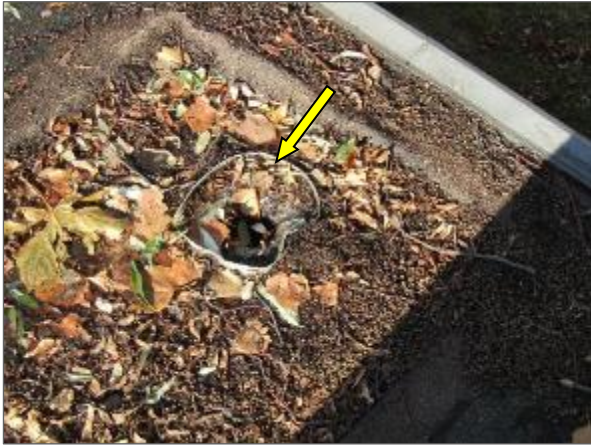
View of a missing roof drain strainer and accumulated organic debris (i.e., leaves) noted at the northwest portion of the modified bitumen roof system serving the Phase 2 portion of the Site Building.
