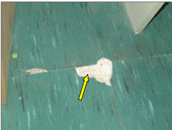
View of deteriorated vinyl floor tile noted within a basement level classroom in the Phase 2 portion of the Site Building.
