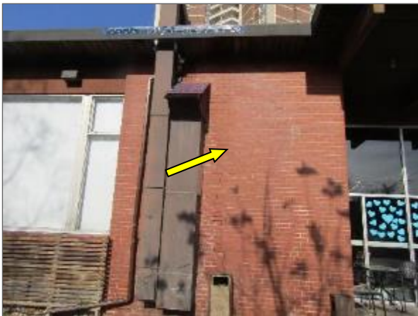
View of the efflorescence stained brick masonry noted on the south elevation of the Phase 2 portion of the Site Building.
