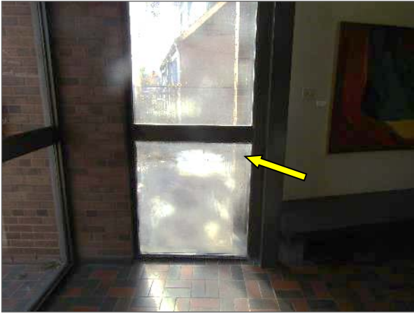
View of the failed IG window unit noted on the south elevation of the Phase 3 portion of the Site Building.
