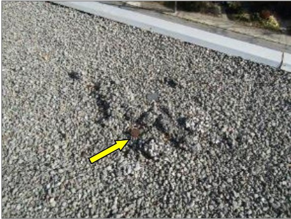
View of asphalt bleed-through noted at the east portion of the BUR system serving the Phase 3 portion of the Site Building.
