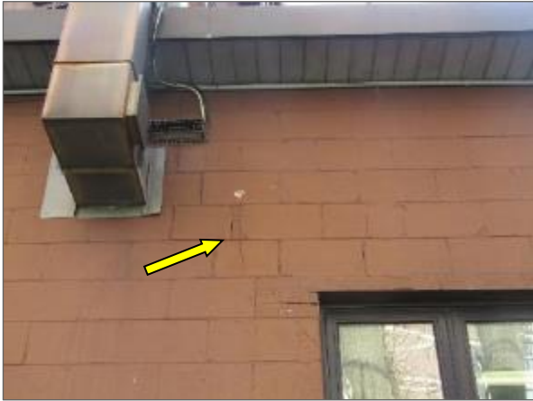
View of step cracking on the concrete block masonry wall noted on the north elevation of the Phase 2 portion of the Site Building.
