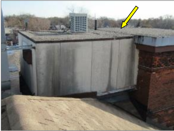
General view of the BUR mechanical penthouse noted atop the Phase 1 portion of the Site Building.
