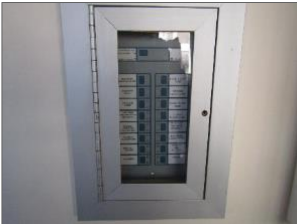
View of the annunciator panel located in the ground floor elevator lobby.
