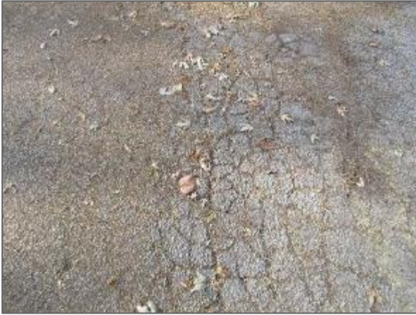
View of alligator cracking in the asphalt pavement noted at the west portion of the Site.
