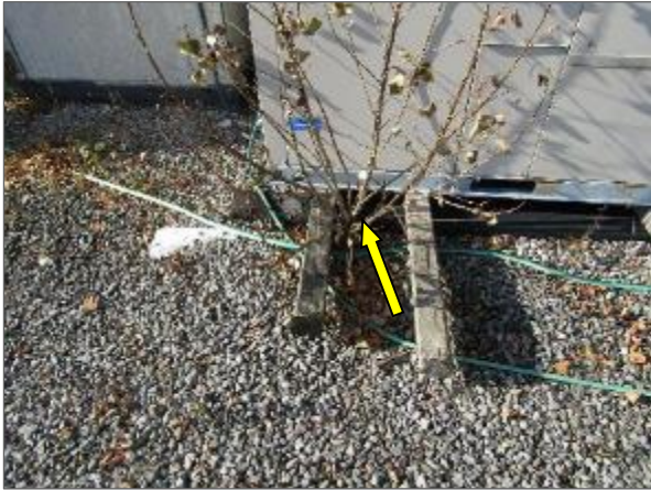
View of the vegetation growth noted at the central portion of the BUR system serving the Phase 3 portion of the Site Building.
