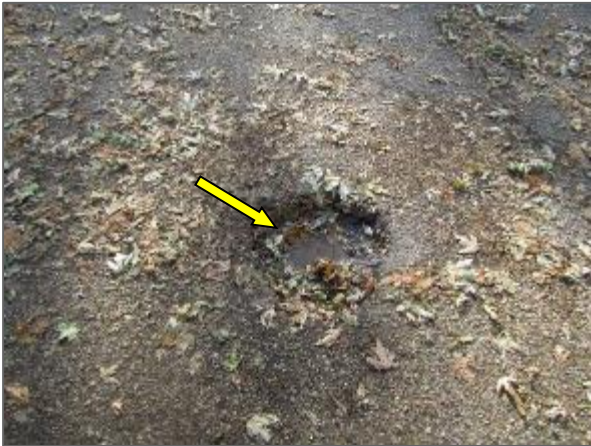
View of alligator cracking in the asphalt paved parking area noted at the west portion of the Site.
