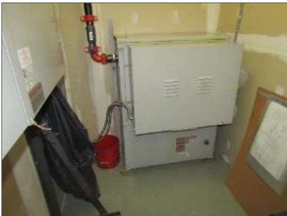
View of the hydraulic elevator system located in the basement elevator room.
