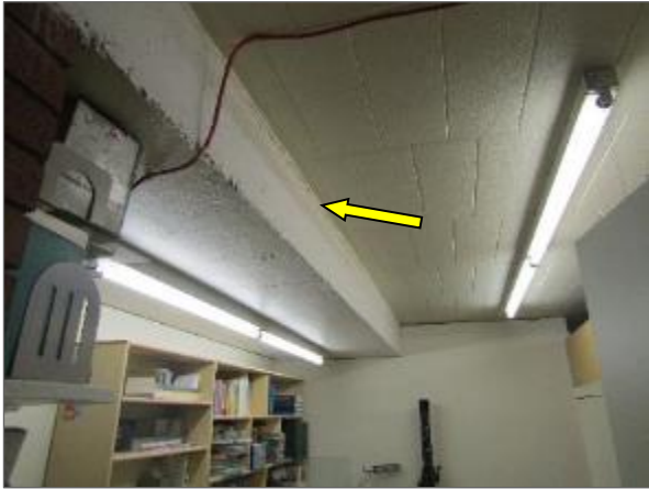
General view of the cast-in-place concrete beam noted within the basement level archive room of the Phase 3 portion of the Site Building.
