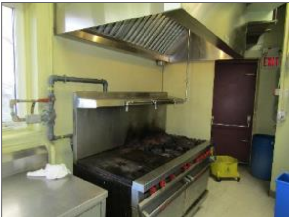
View of the fire suppression equipment noted above the cooking ranges.
