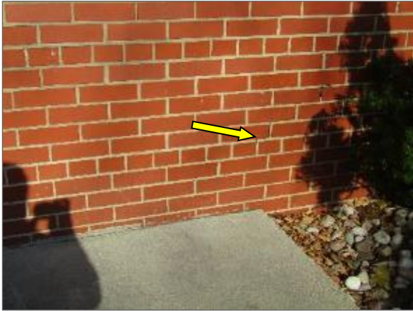
View of the step cracking on the brick masonry wall noted on the south elevation of the Phase 2 portion of the Site Building.
