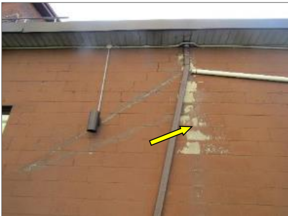
View of moisture damaged/spalled concrete block masonry noted on the north elevation of the Phase 2 portion of the Site Building.
