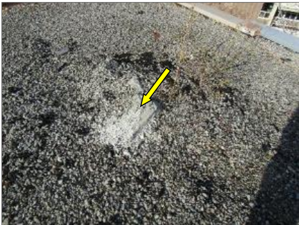
View of a cement deposit (i.e., used as a temporary leak repair) at the northeast portion of the BUR system serving the Phase 3 portion of the Site Building.
