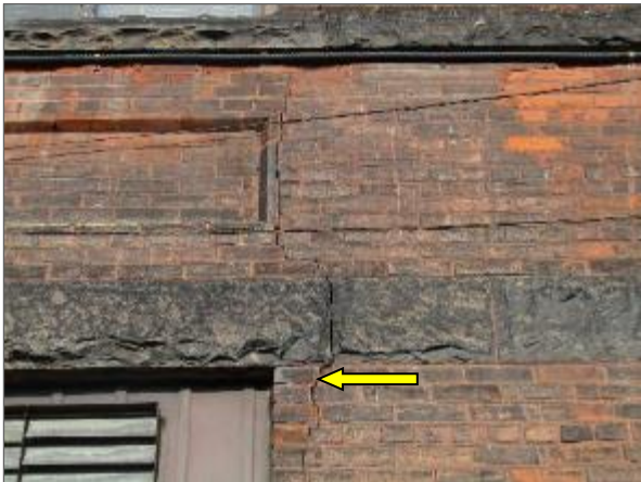
View of vertical/step cracking in the multi-wythe brick masonry wall noted on the south elevation of the Phase 1 portion of the Site Building.
