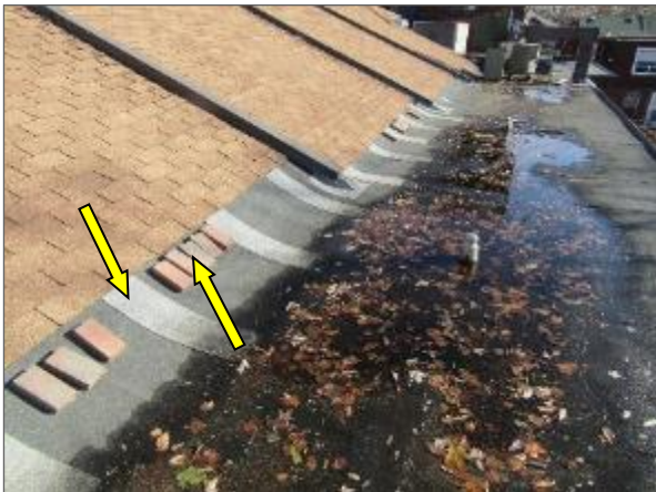
View of the previous patch repairs and debris (i.e., bricks) noted at the south portion of the modified bitumen roof system serving the Phase 2 portion of the Site Building.
