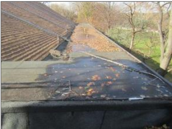
General view of the modified bitumen roof system noted at the perimeters of the Phase 2 portion of the Site Building.
