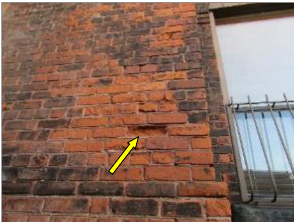
View of the spalled multi-wythe brick masonry noted on the west elevation of the Phase 1 portion of the Site Building.
