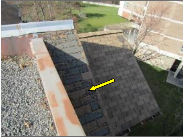
View of the deteriorated asphalt shingles noted at the north portion of the Phase 1, sloped asphalt shingled roof system.
