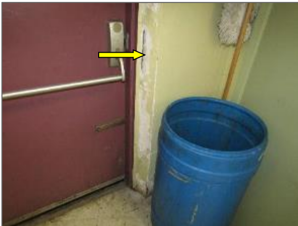
View of the moisture damaged gypsum wall noted within the kitchen area of the Phase 2 portion of the Site Building.
