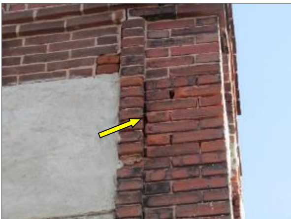
View of the missing mortar joints multi-wythe brick masonry noted on the west elevation of the Phase 1 portion of the Site Building.
