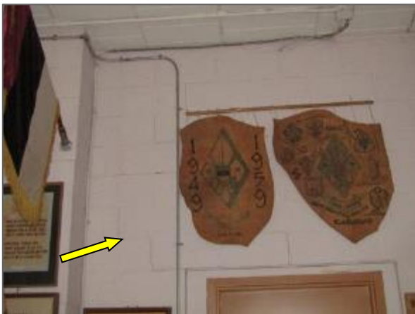
View of step cracking on the concrete block masonry wall noted within the youth room located in the Phase 3 portion of the Site Building.
