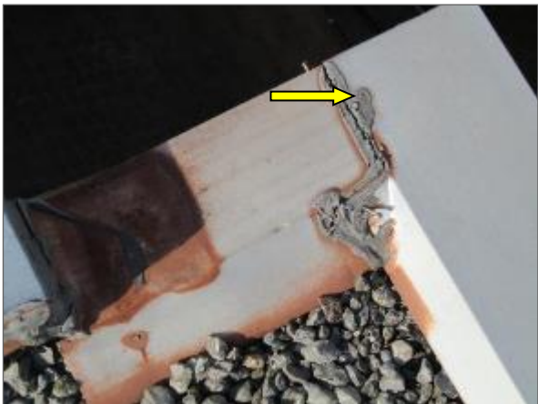
View of a cracked joint sealant serving the perimeter metal flashing serving the phase 3 portion of the Site Building.
