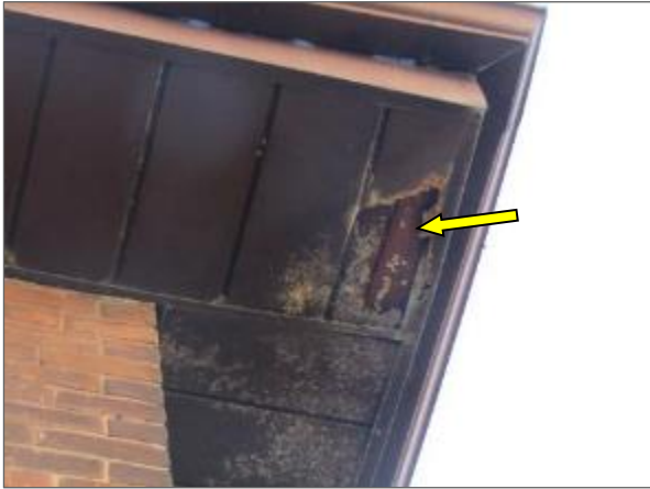
View of the corroded metal soffit noted at the southwest corner of the Phase 1 portion of the Site Building.
