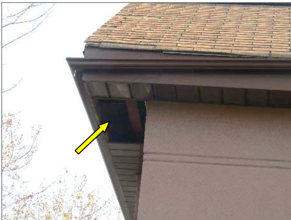
View of missing metal panels serving the soffit noted at the northwest corner of the Phase 1 portion of the Site Building.
