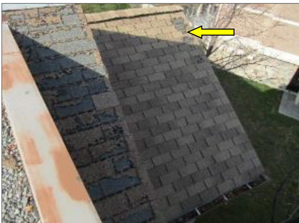
General view of the upper sloped asphalt-shingled roof system serving the Phase 4 (i.e., northeast) portion of the Site Building.
